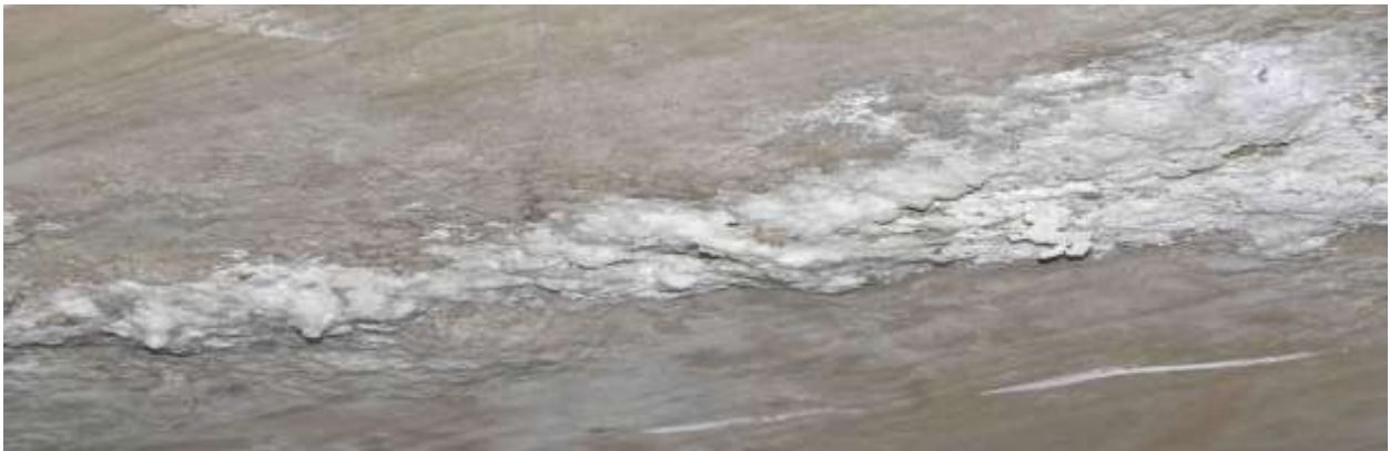
Fig 2 : Example of secondary efflorescence in parking garage exposed to diluted road salt from vehicles entering the garage during winter.
