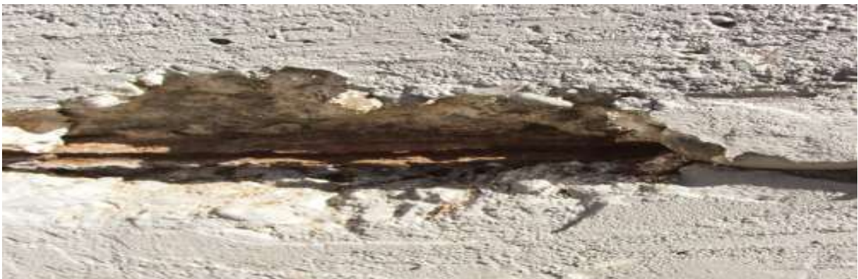
Fig 3 : Spalling due to rusting rebar.
