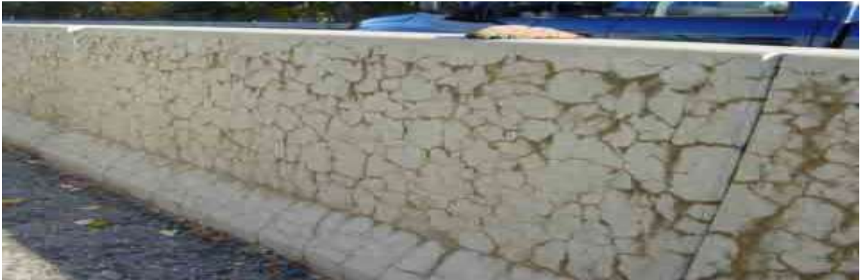
Fig 1 : Example of flat piece of concrete having dislodged with corroded rebar underneath, Welland River bridge across Queen Elizabeth Way in Niagara Falls, Ontario.
